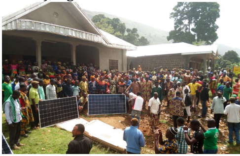
Villagers from Abuk, Cameroon gather as PV panels and other equipment is unloaded and electrification of the community center begins.
